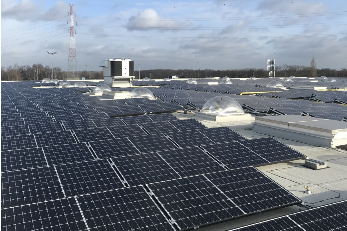
Solar panel array at Decathlon Kuringen
